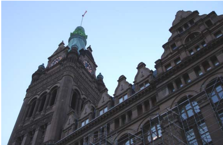
Figure 2. Once a prime example of late 19th Century natural cement architectural construction, Milwaukee City Hall's use of portland cement in restoration has practically eradicated the record of the unique construction technology originally employed.
