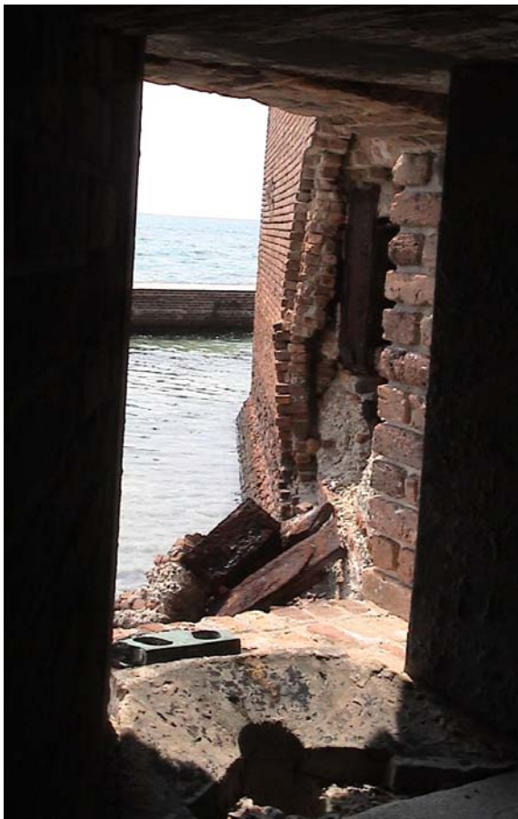
Figure 6. Corrosion of cast iron shutters at Fort Jefferson caused masonry to bow outward more than 12 inches, in some areas. The low modulus/high creep of the natural cement mortar used in original construction accommodated such movement for up to 150 years.
