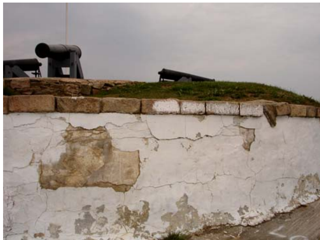
Figure 3. Use of incompatible portland cement stucco at Fort Phoenix accelerated damage to original materials, which were lime-based. The damage took years to develop.
